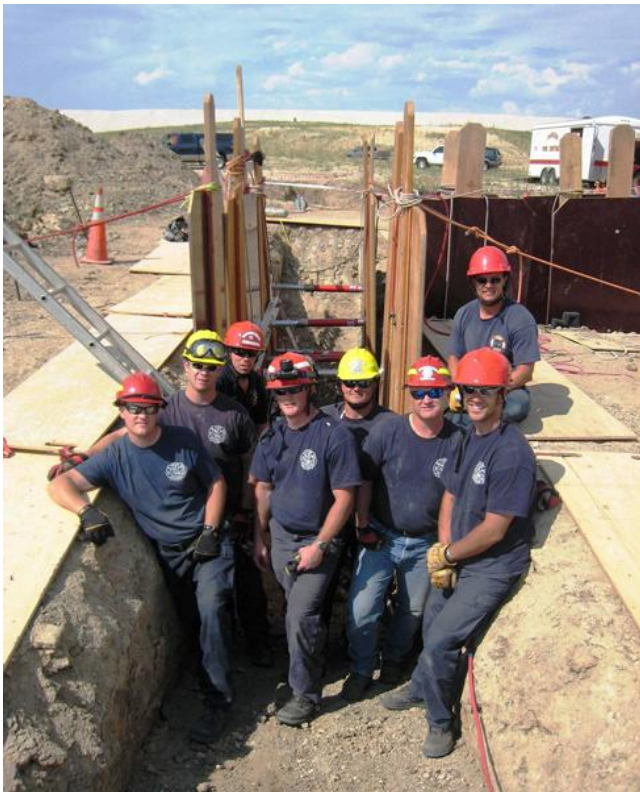
Figure 11-7 Work with your members during training so that you and they know what to expect during incident operations
